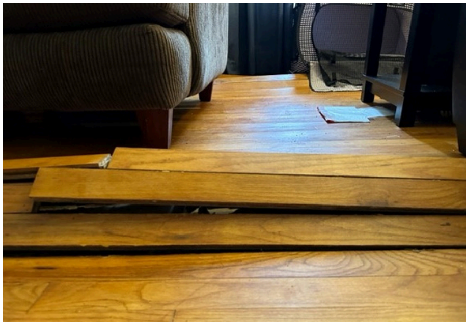
Apartment leak from a water pipe causing damage to floor.
